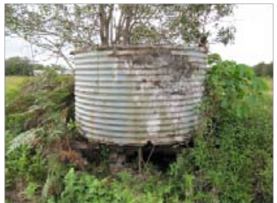
WB H-1. Standing rainwater tank on wooden posts and more recent brick piers
